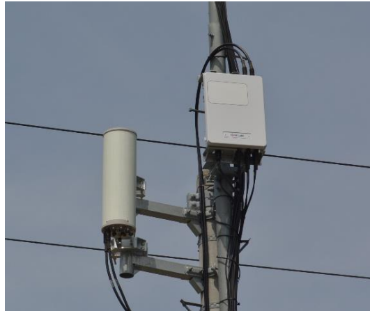
Relay Node Station
